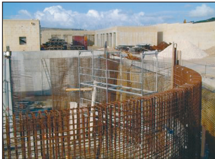
Construction of the Malta North Sewage Treatment Plant. Will the south keep up?
